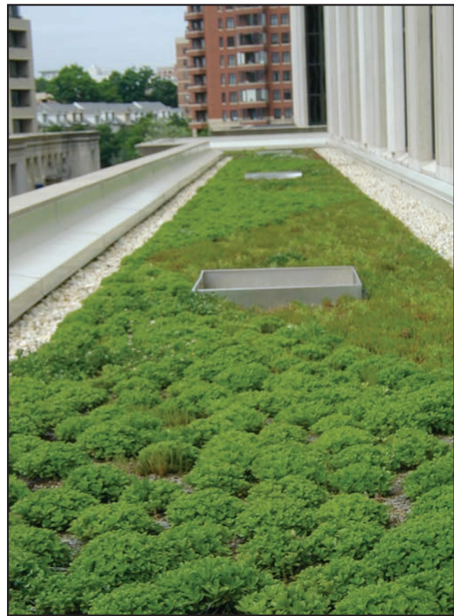
Figure 41. This green roof constructed on top of a building acts as a bioretention system. (Photo courtesy of Joan Kelsch, Arlington County Government.)
